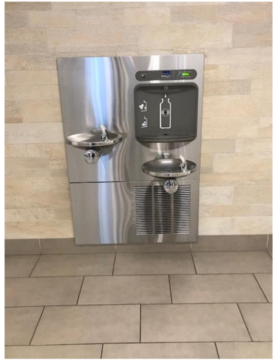
Figure D-17: Water bottle filling station within terminal building.
